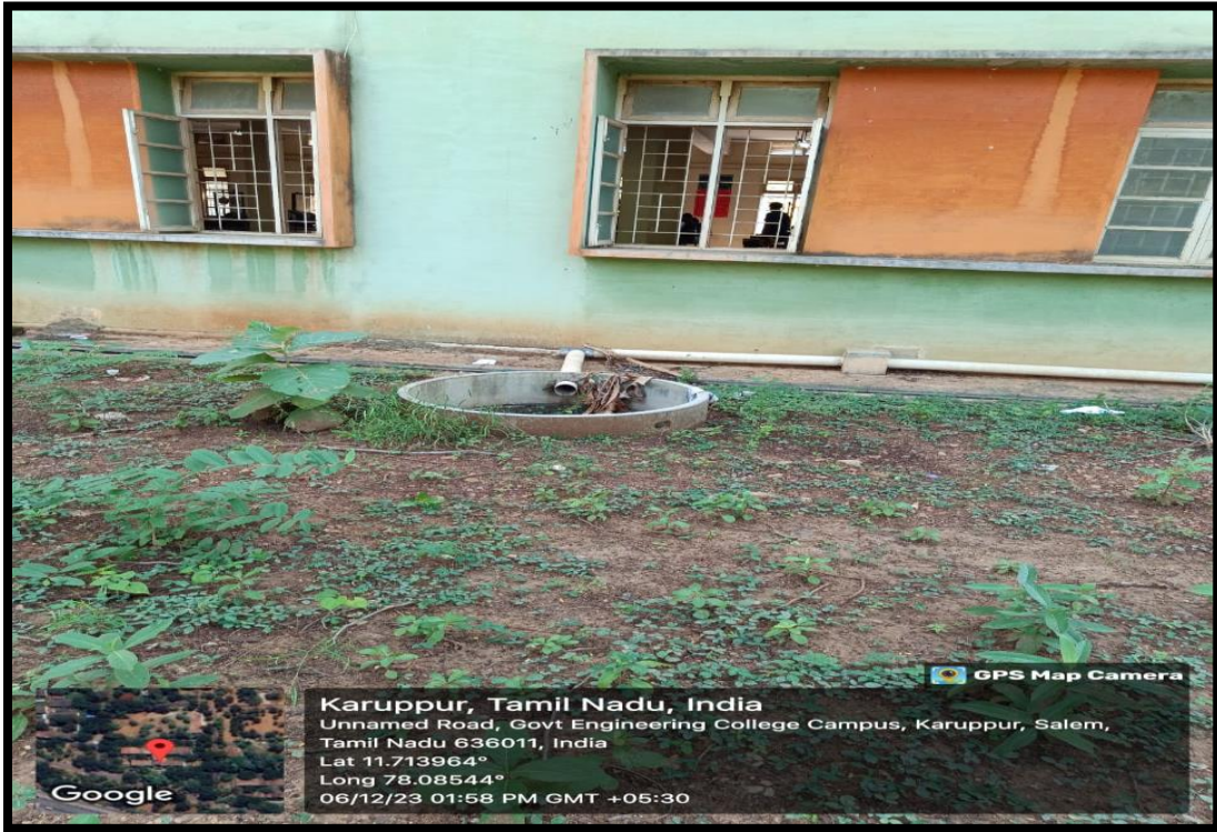
Figure 4: Rainwater harvesting Pit in Department of EEE
