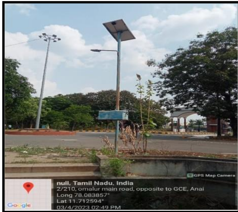
Figure 1: Solar energy-based street lighting system
