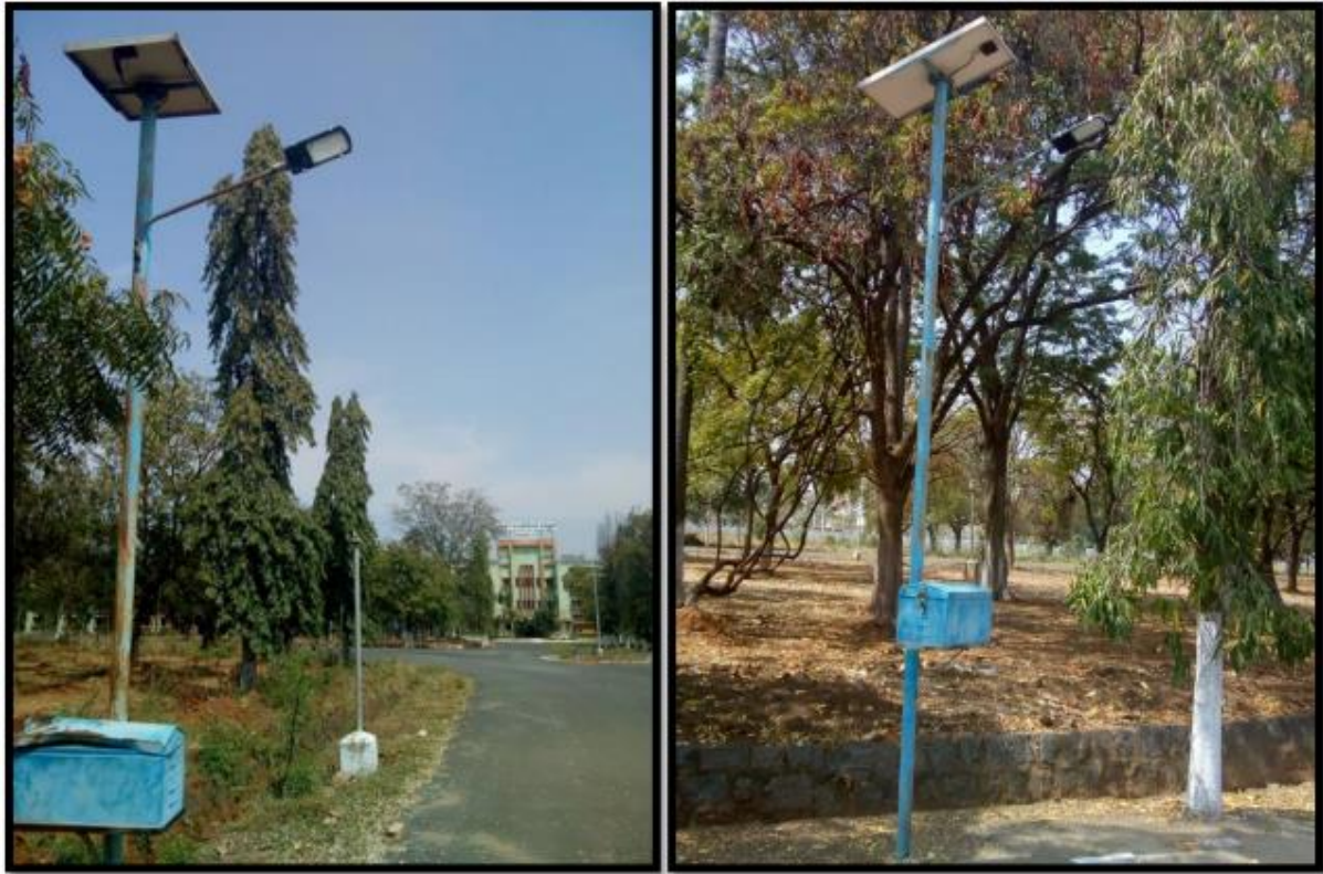
Figure 3: Solar energy-based street lighting system
