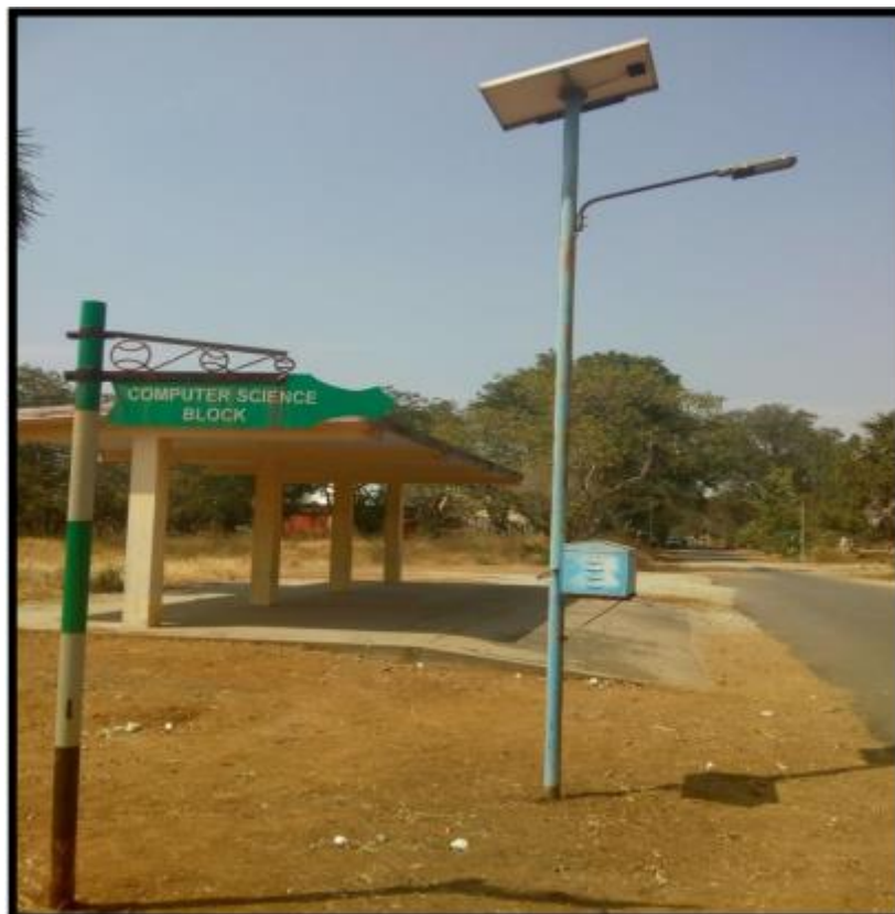
Figure 2: Solar energy-based street lighting system
