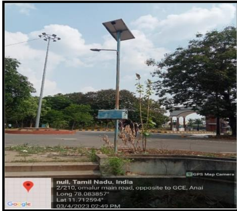
Figure 1: Solar energy-based street lighting system
